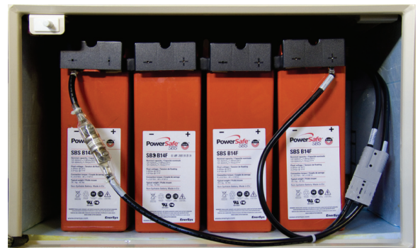
Fig. 2-19, Example of Completed Battery Installation
